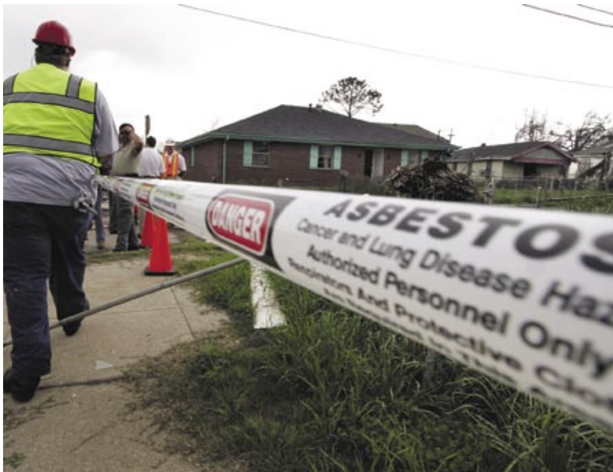
AN ASBESTOS caution tape is wrapped around the site of the demolition of a home in the Lower Ninth Ward of New Orleans in 2006. Asbestos claims overall are down in number, but pockets of severity remain.
